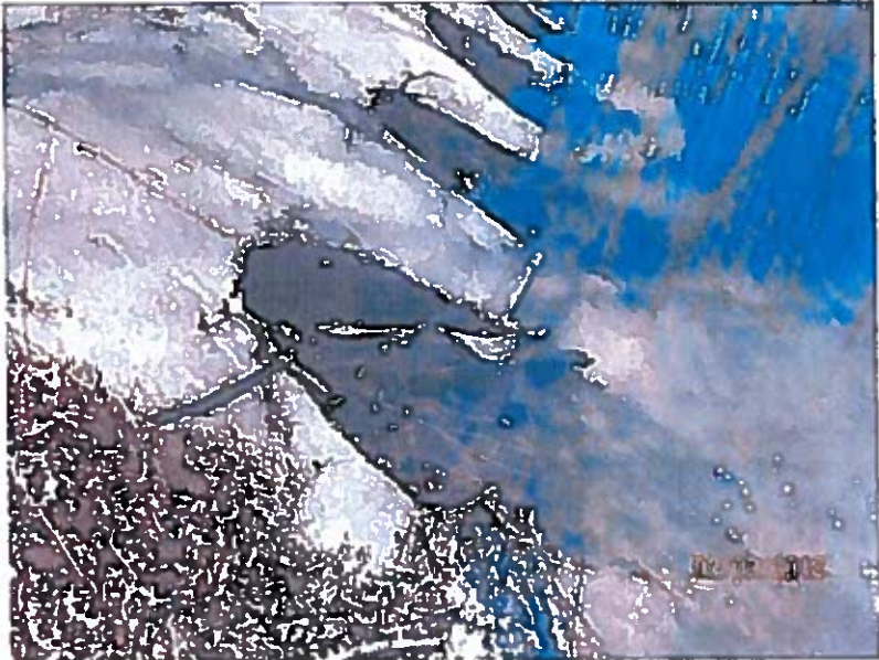
Debris at the inlet of Pipe 1.
