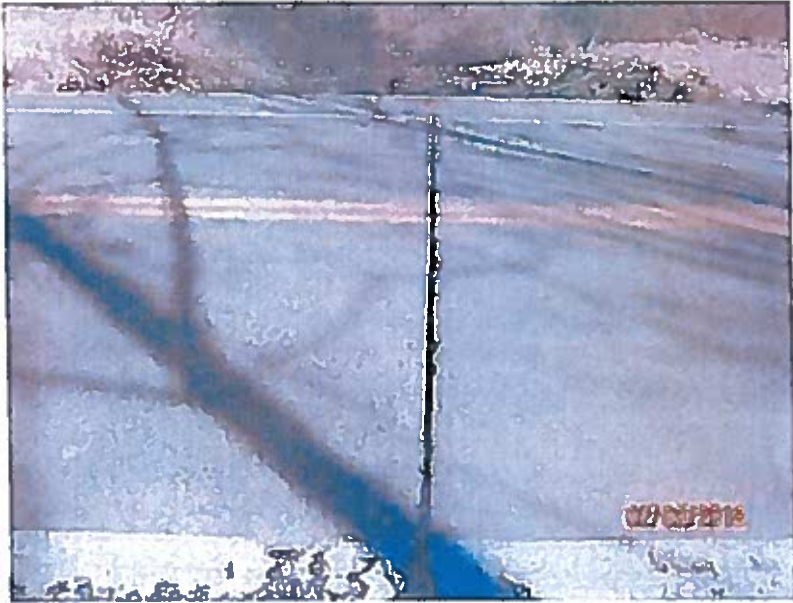
Joint between reinforced concrete slab over pipes and general condition of slab.
